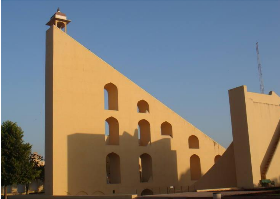
Caption: Brihat Samrat Yantra – with repaired plaster and lime wash (khamira) © DRONAH
